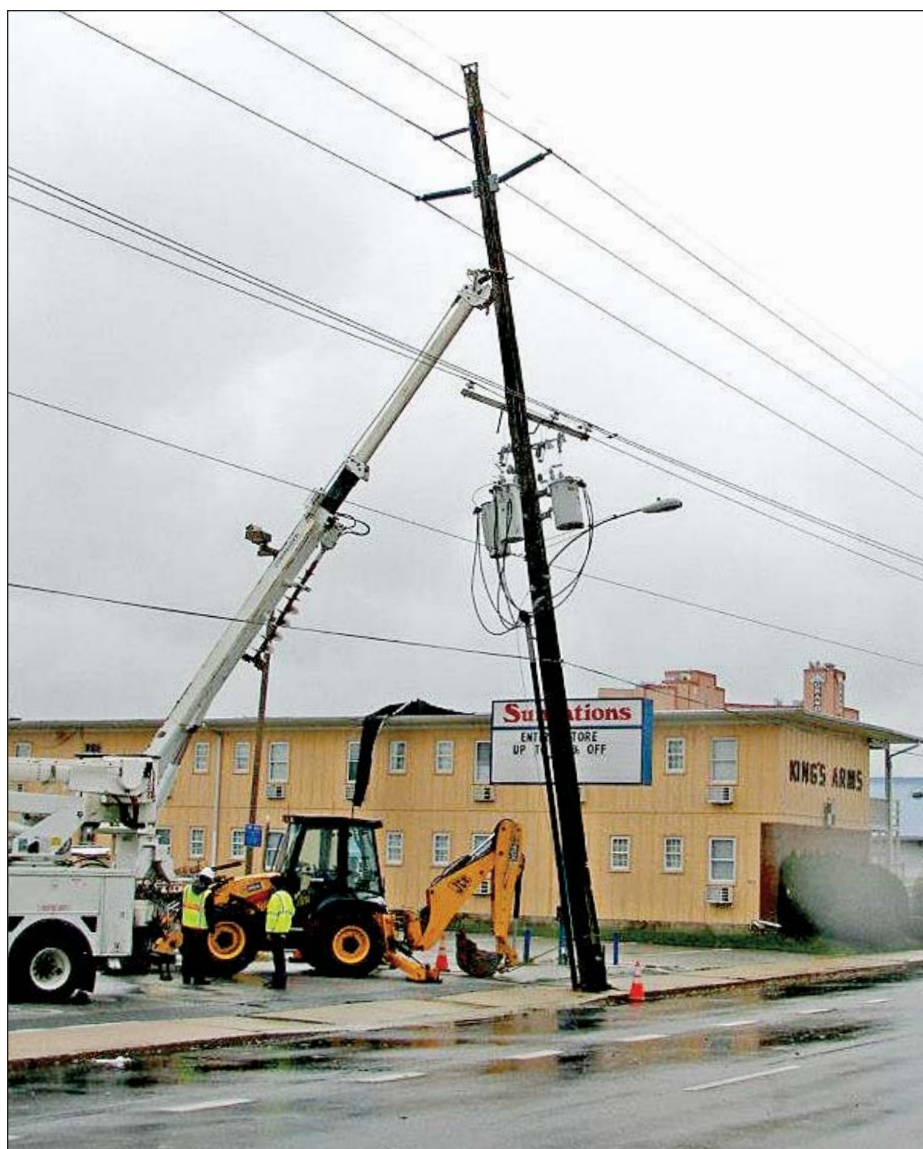
CREWS REPAIR DAMAGE AFTER SANDY Zack Hoopes/Ocean City Today Crews work to replace a cracked telephone pole on the east side of Coastal Highway at 24th Street, following high winds last night from Hurricane Sandy.
