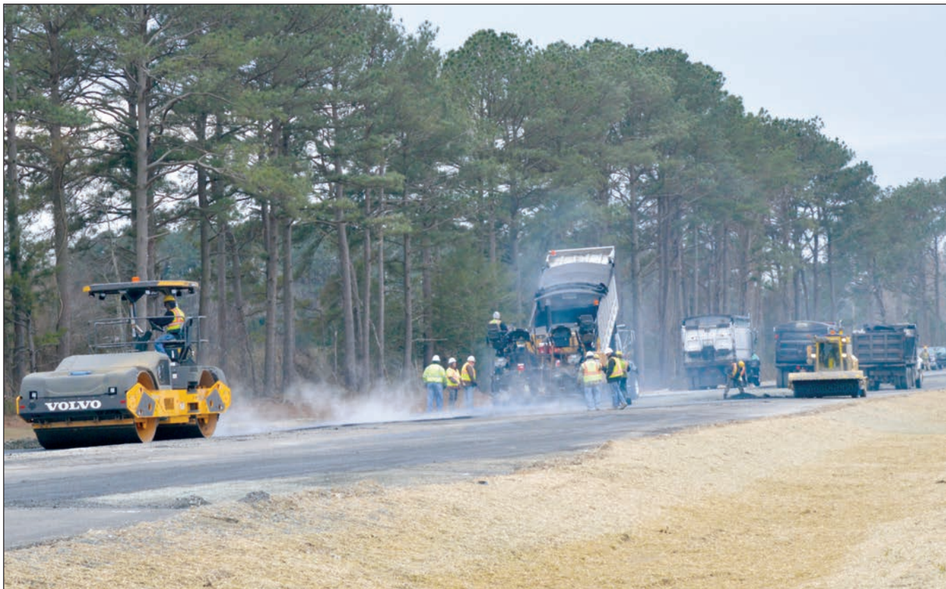
Workers continue dualization work on Route 113, as they pave what will become the new northbound lanes. The State Highway Administration intends to move traffic from the old lanes to the new on Monday.
