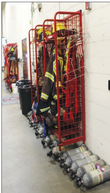
CINDY HOFFMAN/BAYSIDE GAZETTE Storage is an issue at the Ocean Pines South Station. Gear is stored in the Apparatus Bay along with the trucks. A new fire station would provide a decontamination room for gear.
